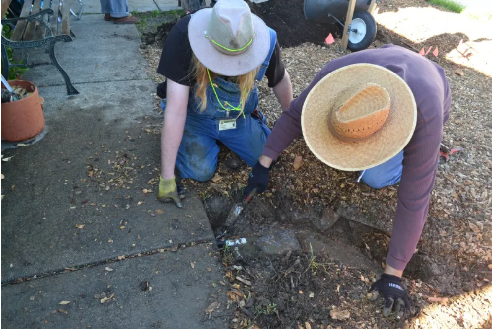
Sustainable Solano project designer Scott Dodson, left, and volunteer Duane Murphy connect a downspout to a swale to catch roof water to pump into the garden in a newly installed food forest in Vacaville. (Nick Sestanovich/The Reporter)
