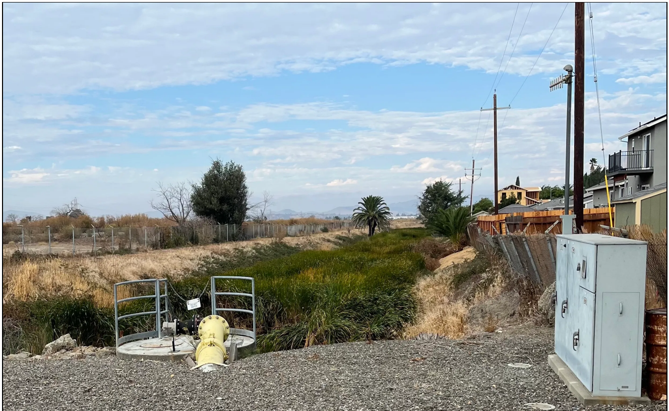
Kellogg pump station. Photo: Aleta George.
